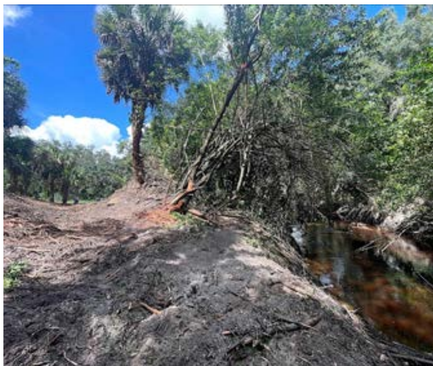
Photo of a breached dike after Hurricane Debby courtesy of Sarasota County
